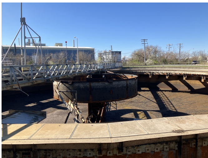
Image 03: Clarifier #6b, empty, bent / twisted skimmer arm.
