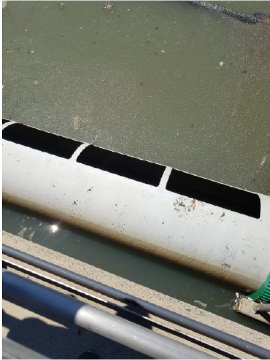
Scum log above water surface 5/6/2021
