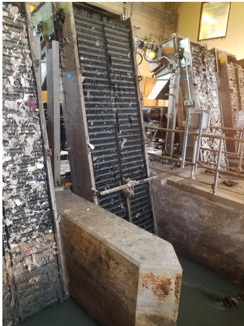
Bar Screens for Fine Screening 5/6/2021
