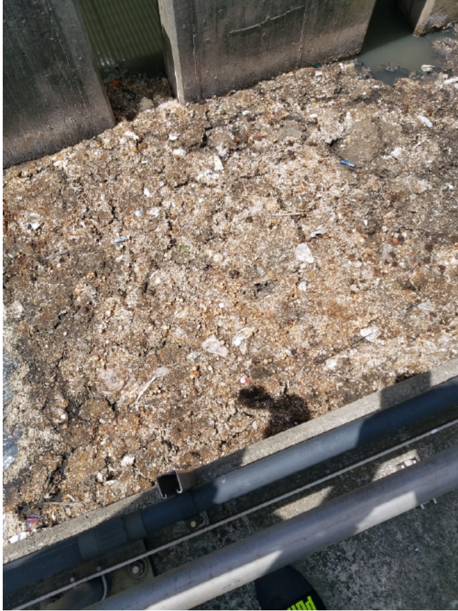
PST Scum trough with excessive amount of FOG 5/6/2021
