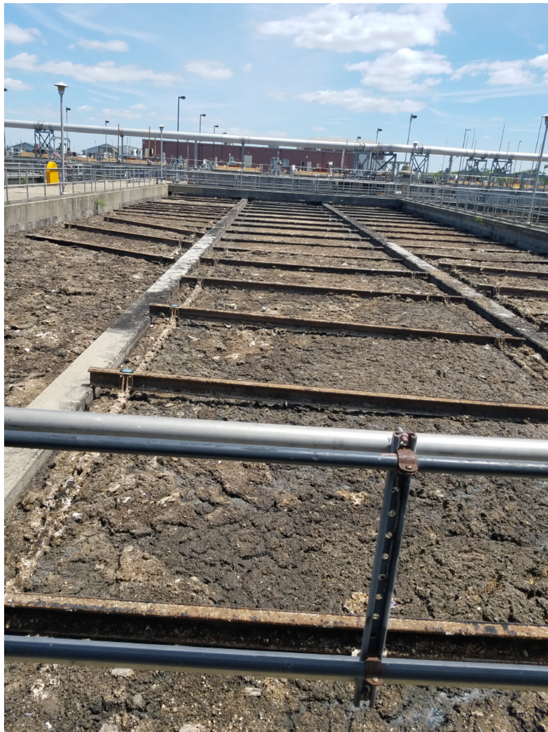
PST not operational due to solids and FOG 5/6/2021
