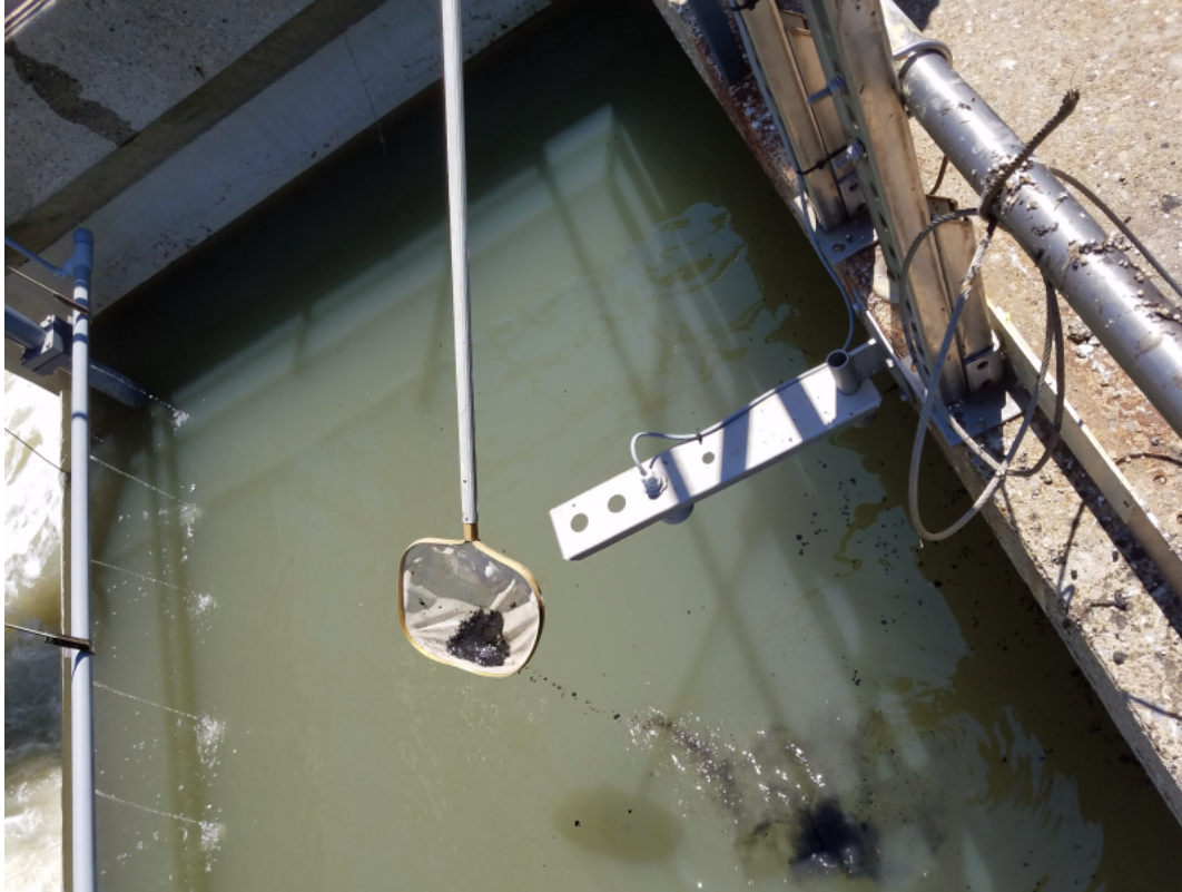
Floating scum being discharged before scum log was lowered 5/6/2021
