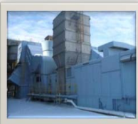
GE Gas turbine
