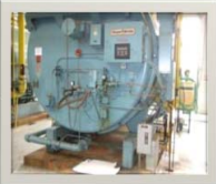
Cleaver Brooks boiler
