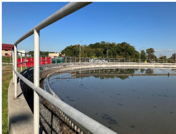
Image 01: PST #11, Missing skimmer.
