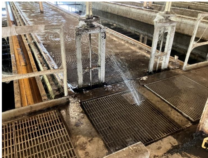
Image 04: Sand Filters, Leak between filters #34 and #36.
