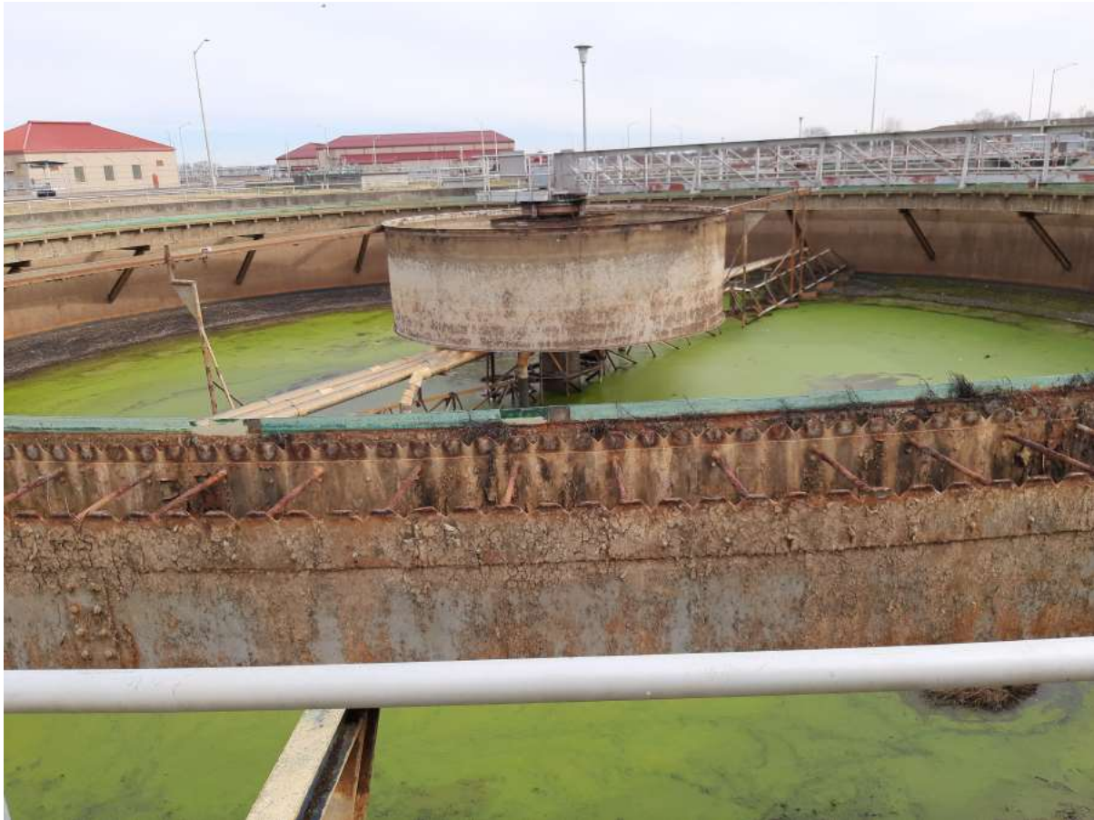
12/14/22 Activated Sludge Plant 3 – Secondary clarifier 16A out of service due to broken mixer
