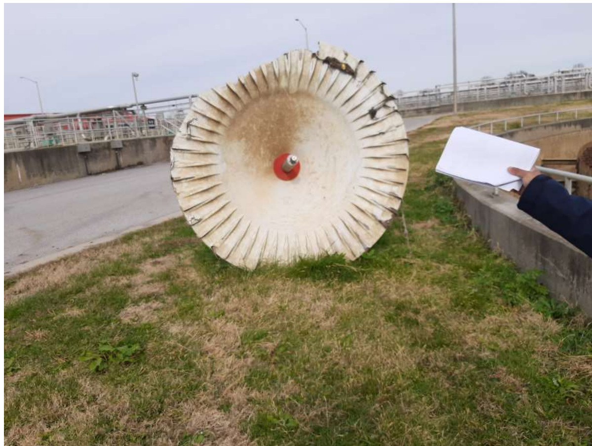
12/14/22 16 A broken mixer- The mixer fell off the assembly and cracked.
