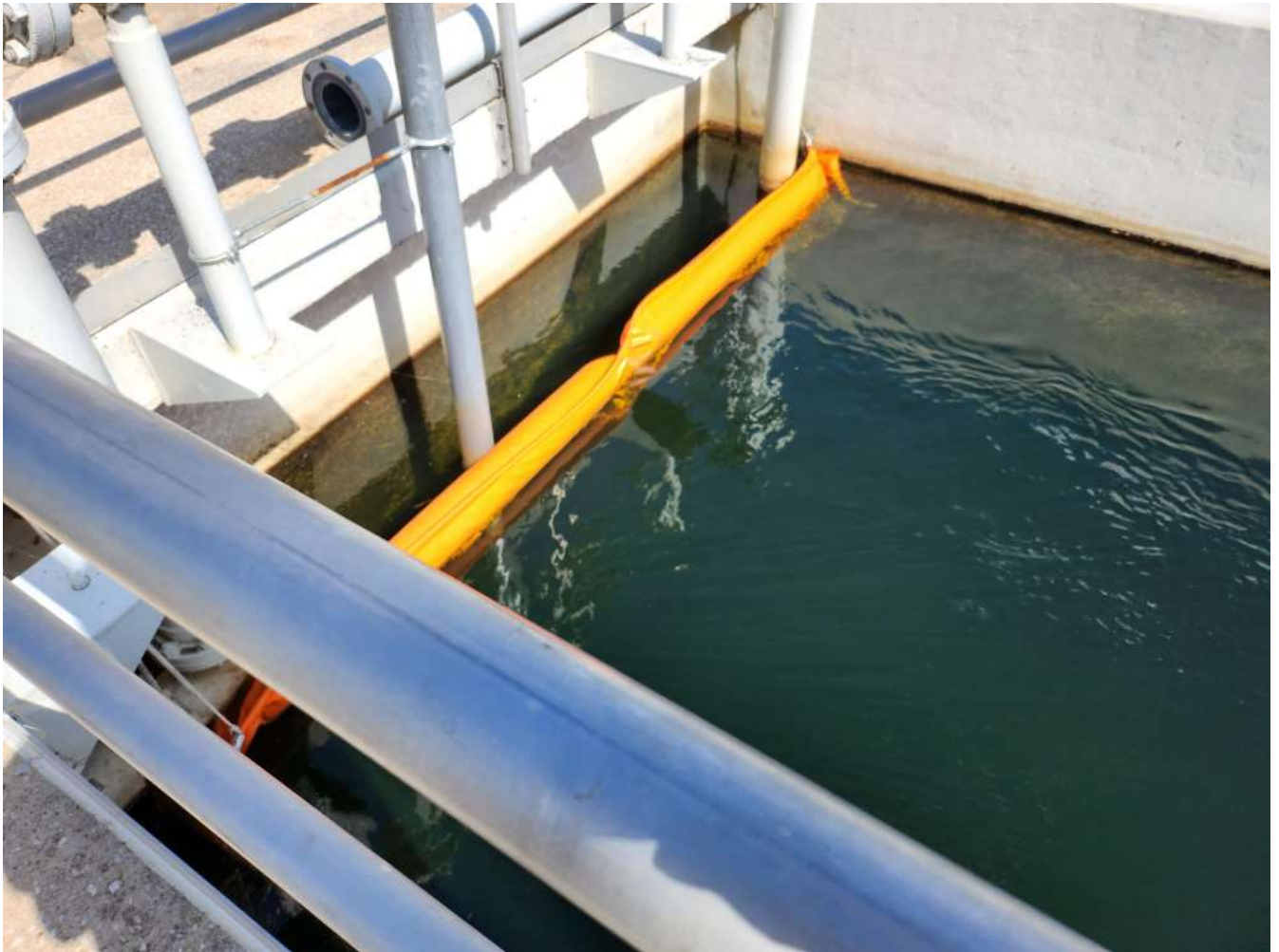
12/14/22 The floating boom at the left channel CCC used to prevent floating solids from entering the final discharge canal.
