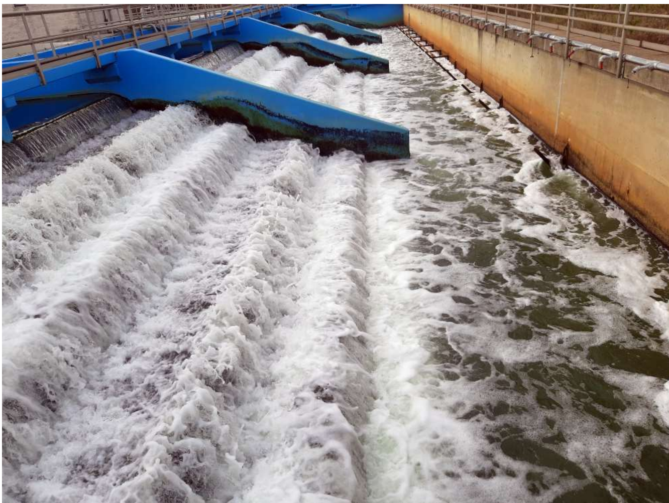
12/14/22 Final effluent at the step aeration discharge configuration
