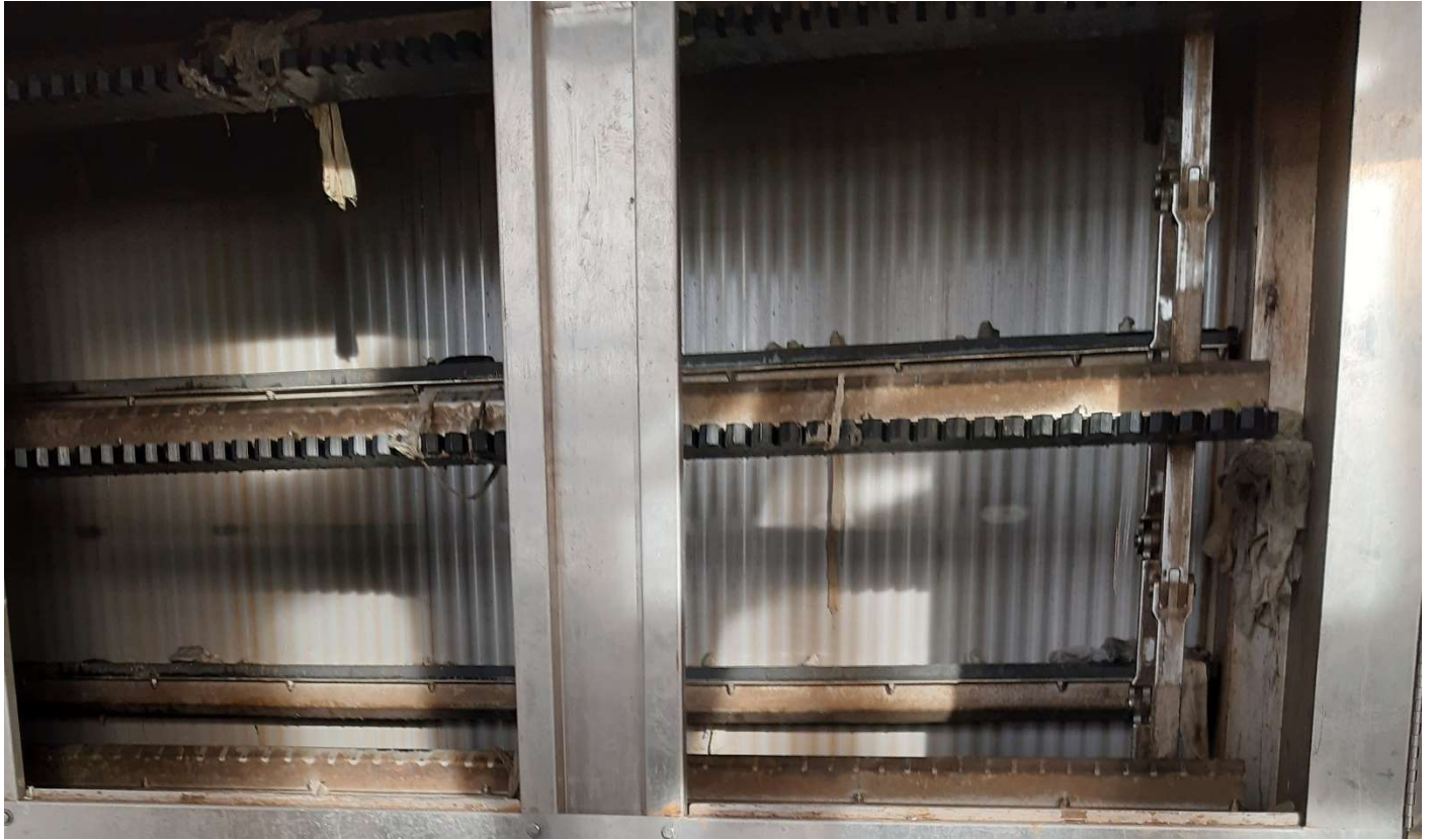
12/14/22 Inside of the functioning coarse screening unit. No problems observed.
