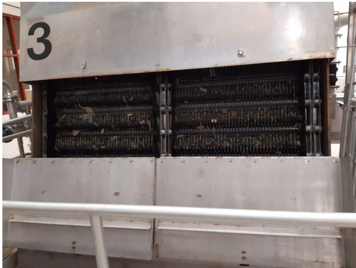
12/14/22 Fine screening unit in service.
