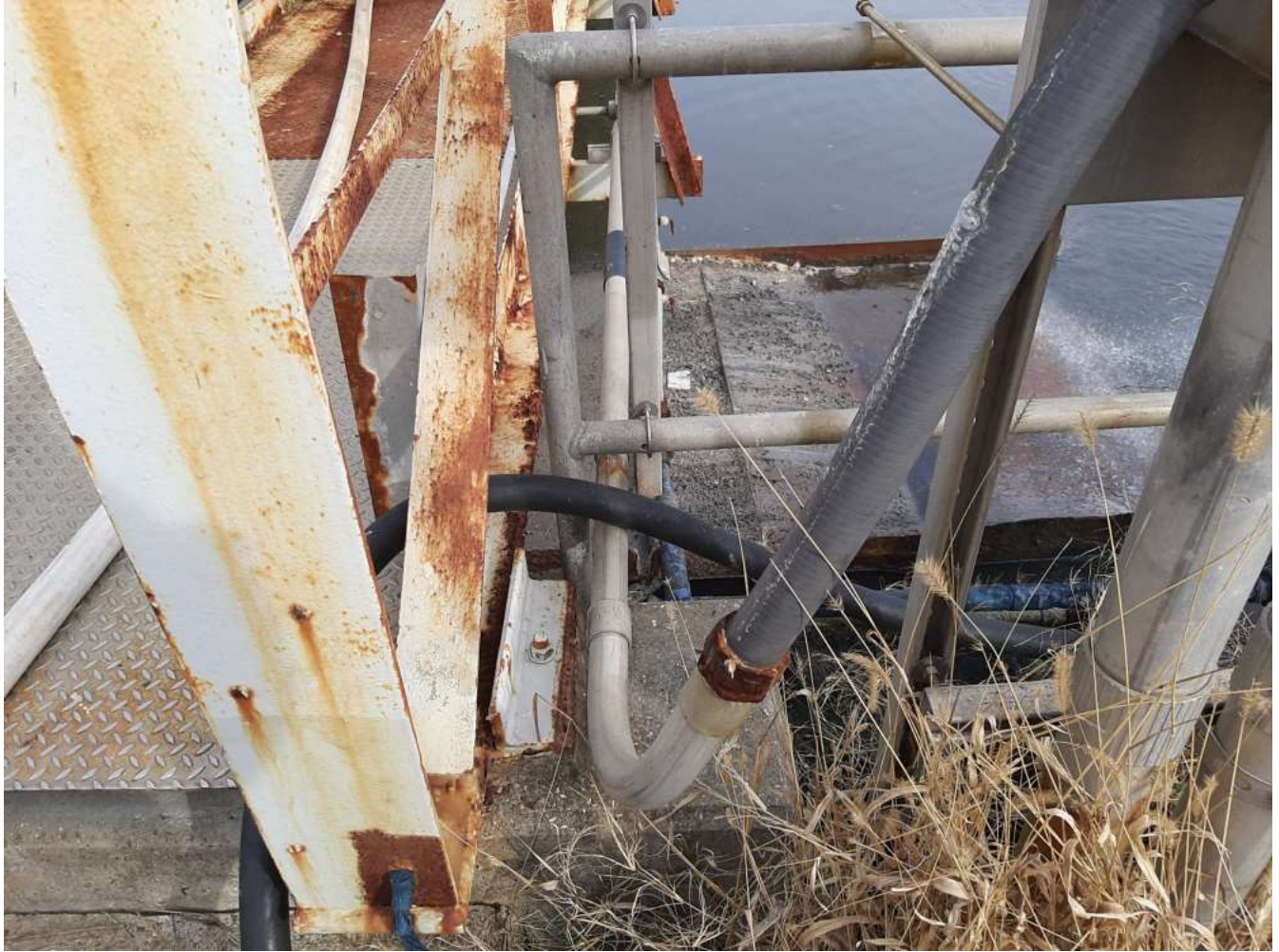
12/14/22 PST #1 scum collection trough clogged. Scum pit requires cleaning
