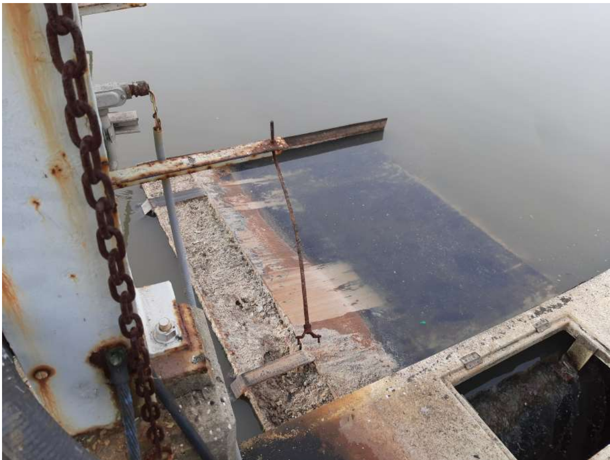
12/14/22 PST #8 scum collection trough filled. The scum pit requires cleaning.
