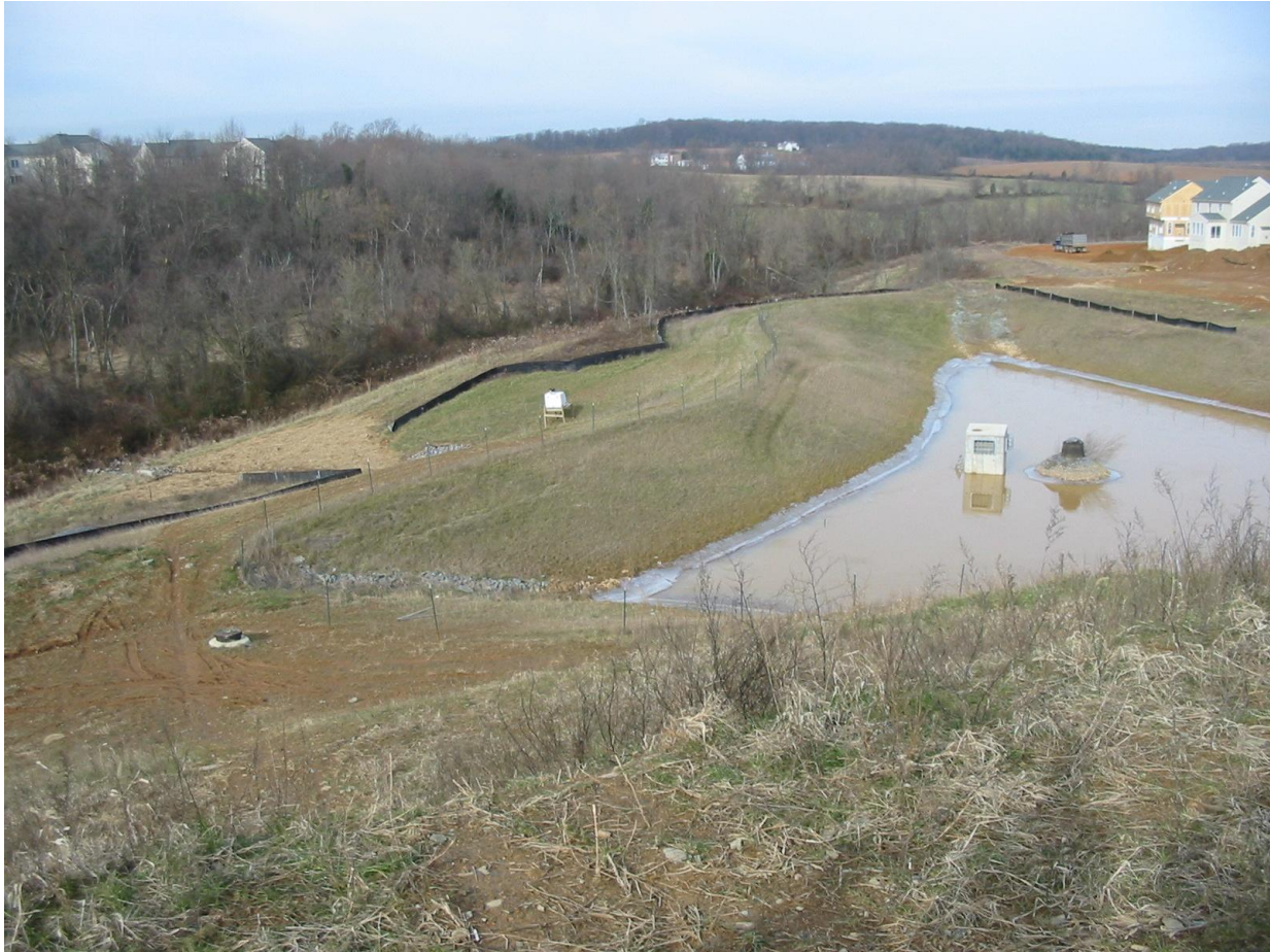
Figure 9a. FRCO's outfall, Pond-R, in December 2002. Storm box containing monitoring and sampling equipment is located in left-center of photo.
