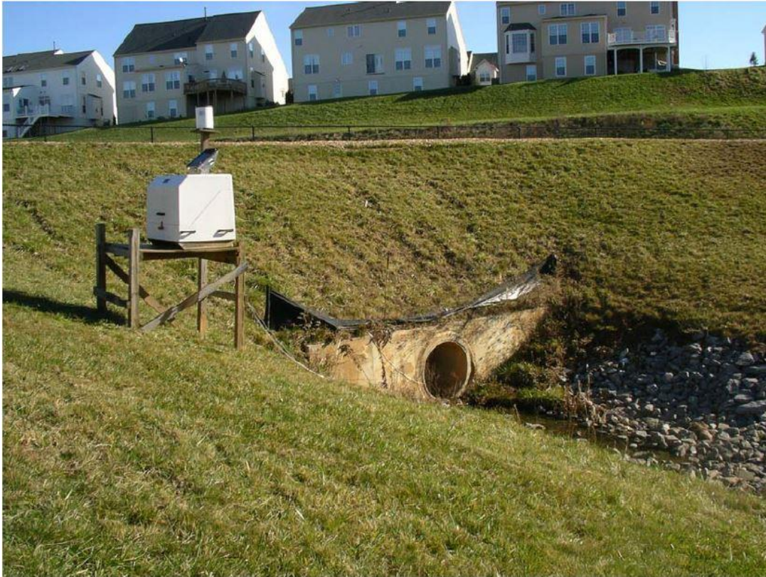
Figure 9b. FRCO's outfall monitoring storm box in December 2004.
