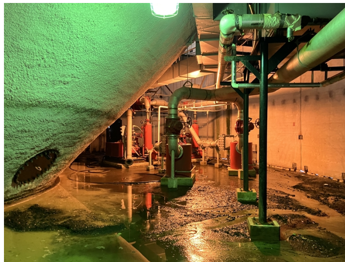
Image 06: Area of the leak below digester #8.
