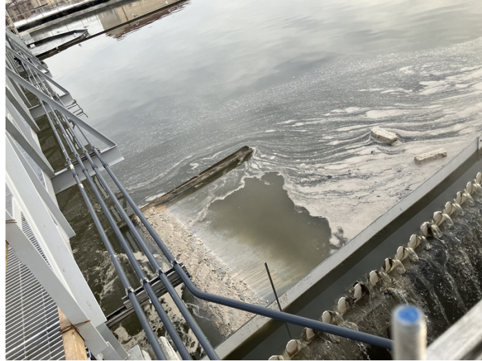
Image 01: PST #10, clogged scum trough.
