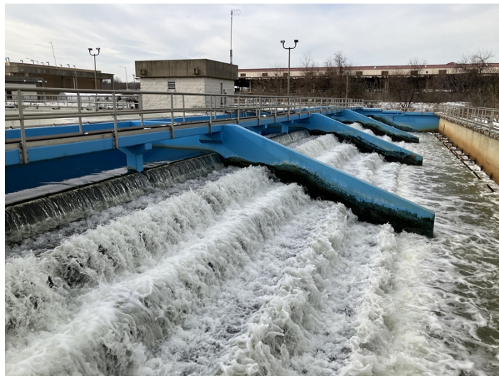
Image 03: Step Aeration system, final effluent.
