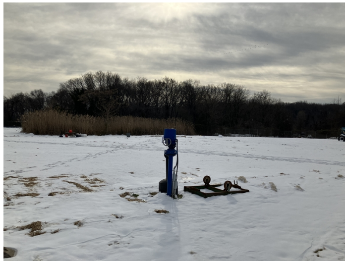
Image 04: Faulty influent flushing water control valve.
