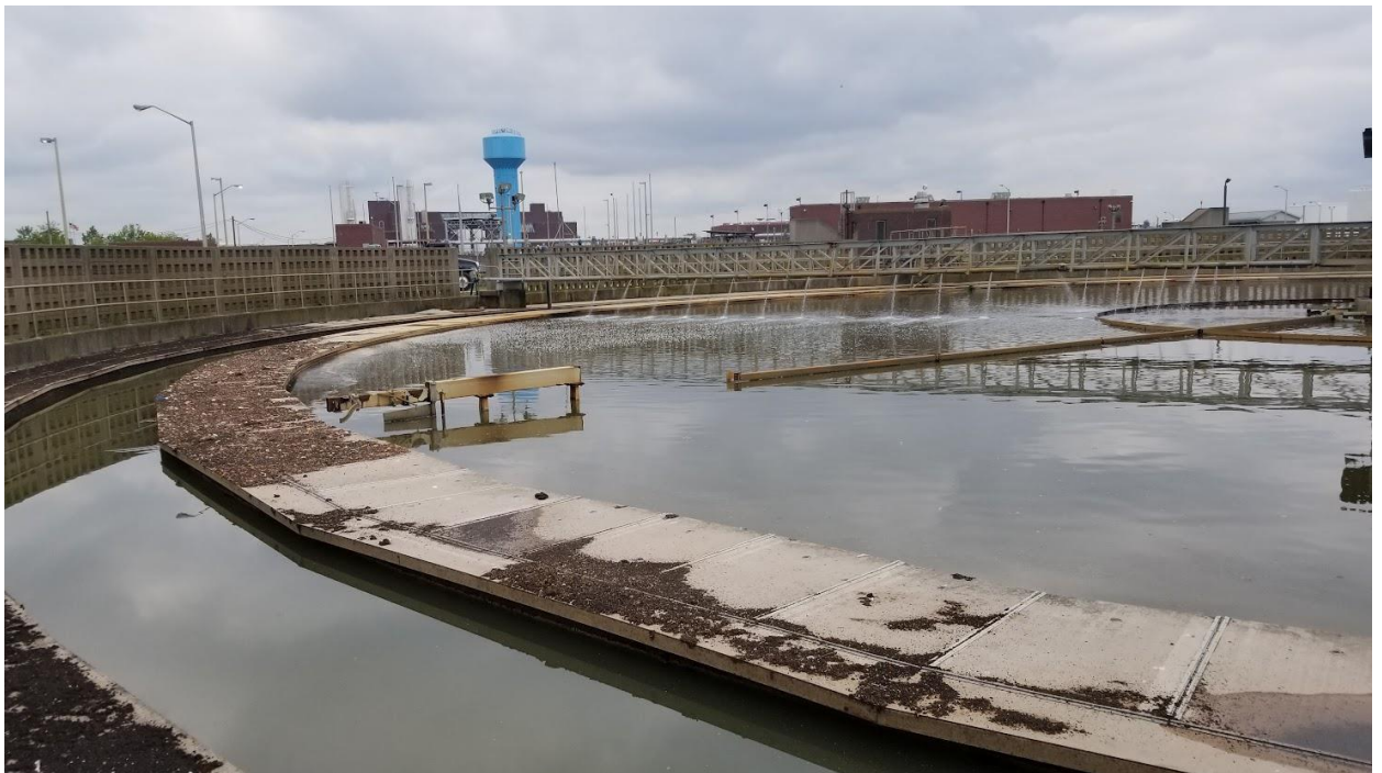
Figure 5d: One of the two scraper arms in Clarifier # 4 is missing.
