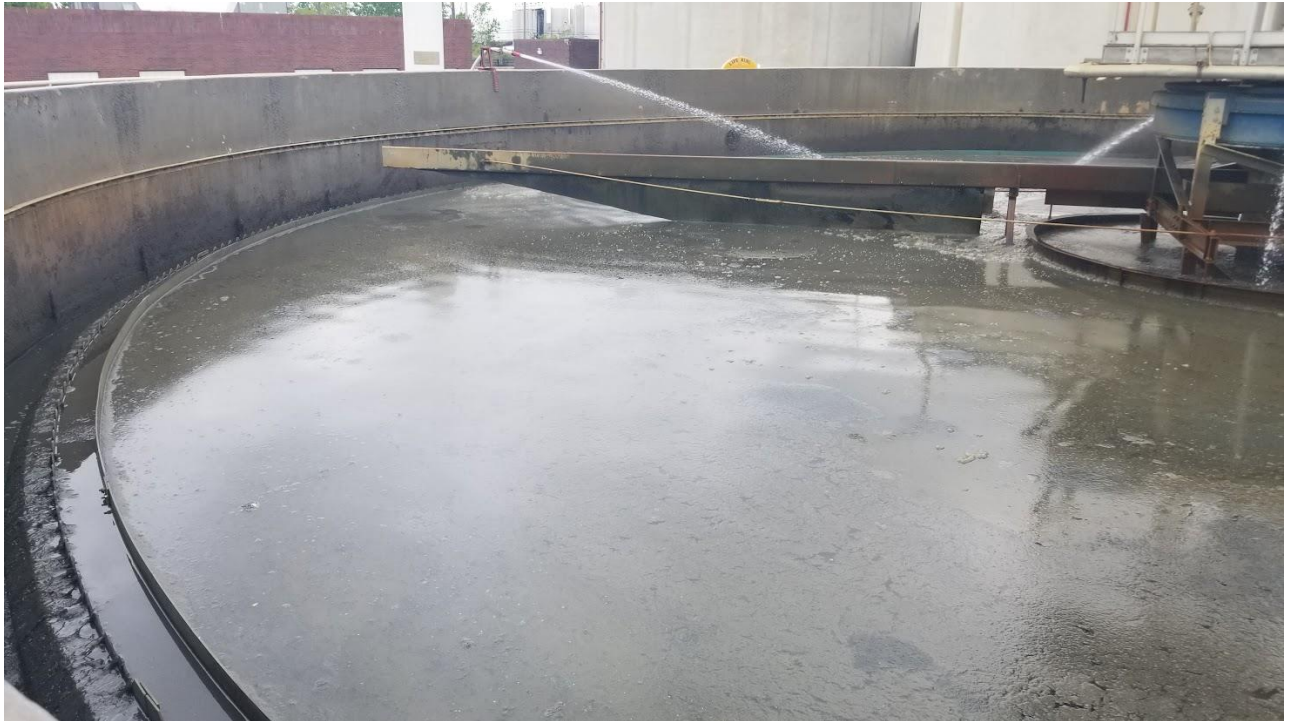
Figure 1c: Sludge at the surface of GST #2. One of the skimmer arms has not been fixed yet and is partially above the water surface level.
