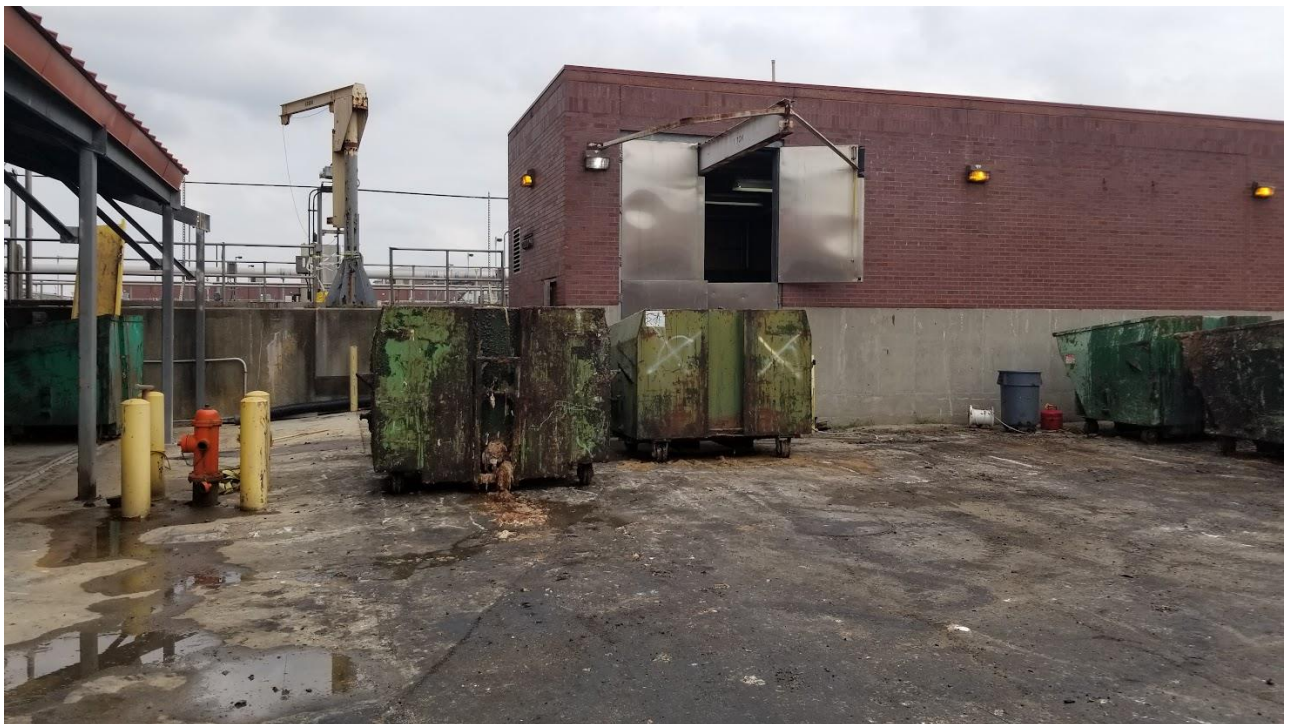
Figure 2b: A leaking hopper by the southwest side of the combined influent building. FOGs are on the ground surface.
