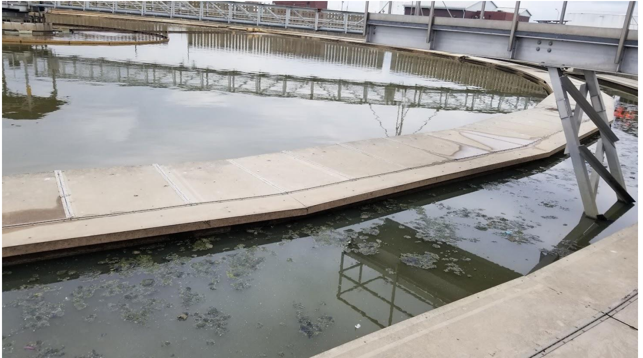
Figure 5c: Algae outside of the launder cover of Clarifier # 4
