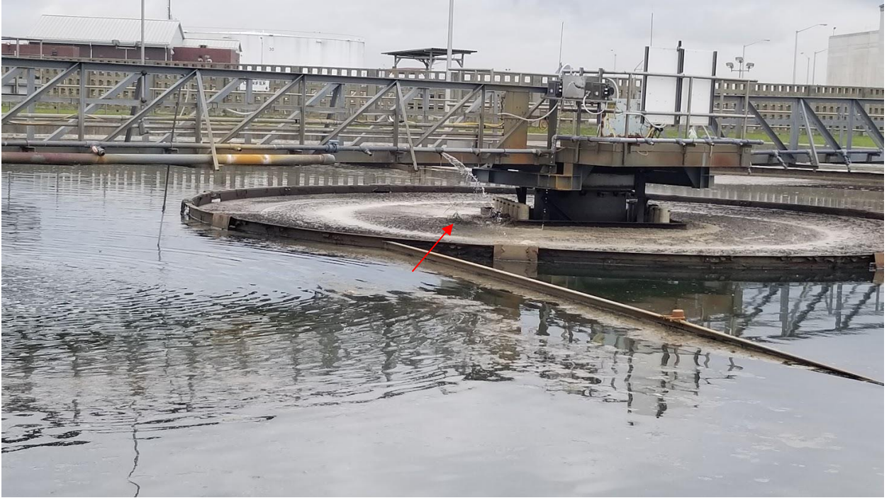
Figure 5i: Grass at the center/ influent side of Clarifier # 5A (pointed to with a red arrow)
