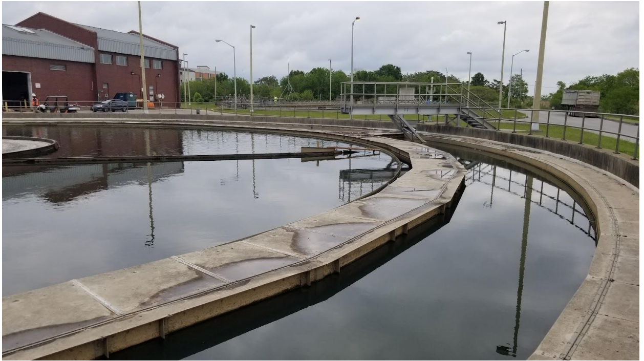
Figure 5g: One of the scraper arms in Clarifier # 6B is missing.
