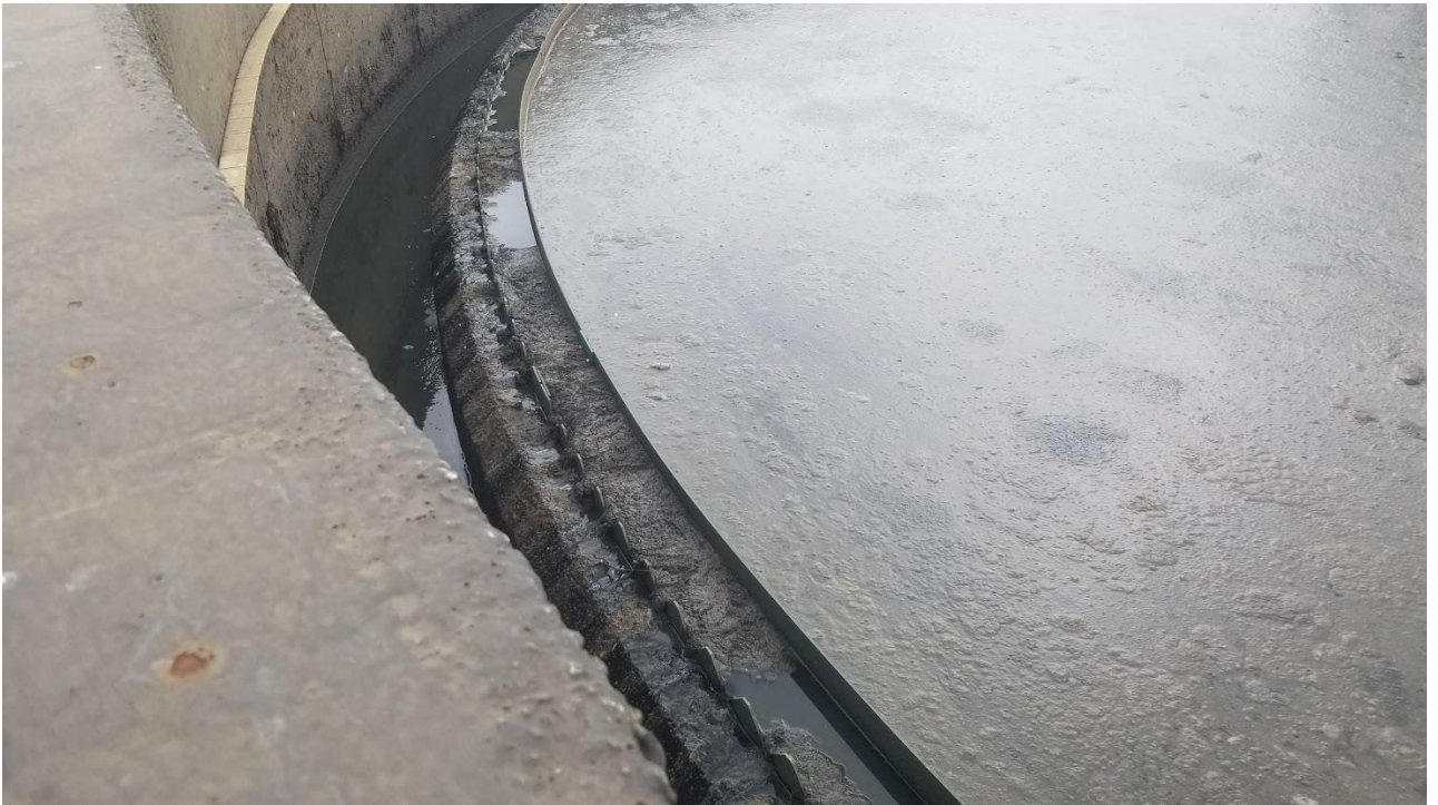
Figure 1b: Close up view of sludge next to the V- notch weir within GST #1.
