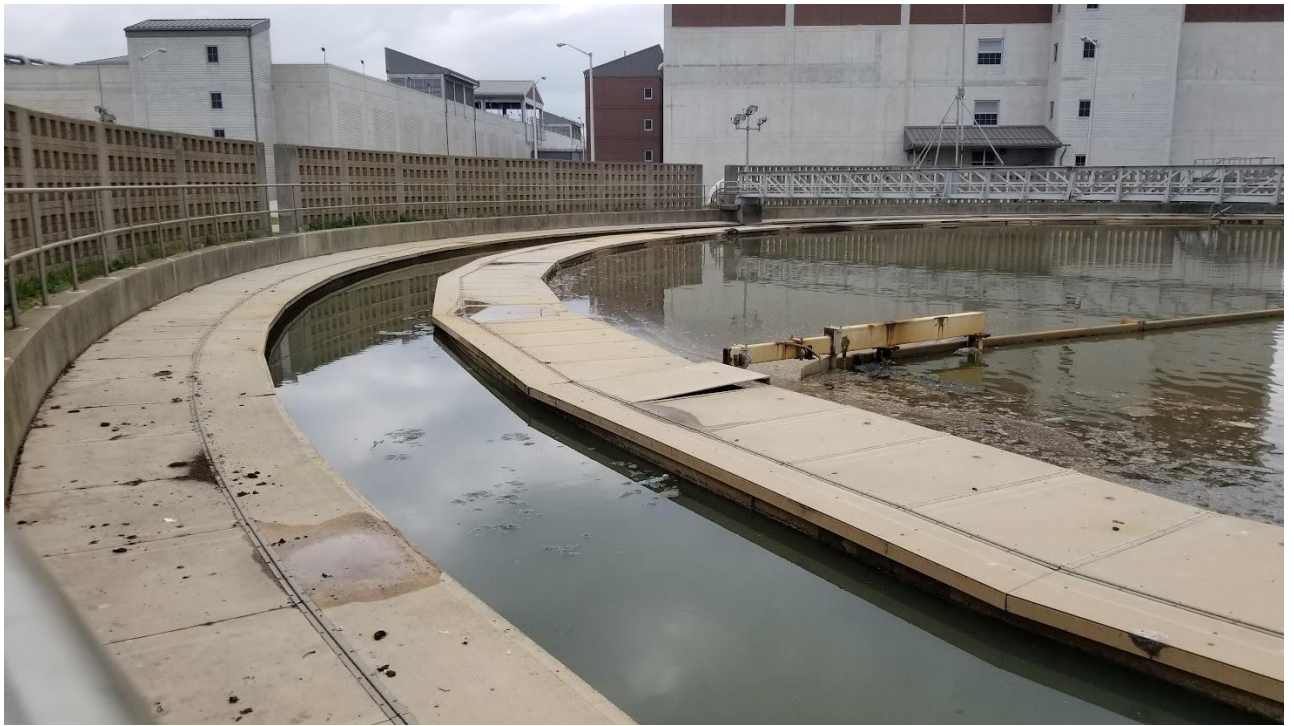
Figure 5b: Rubber piece missing at the edge of one of the scraper arms in Clarifier # 4
