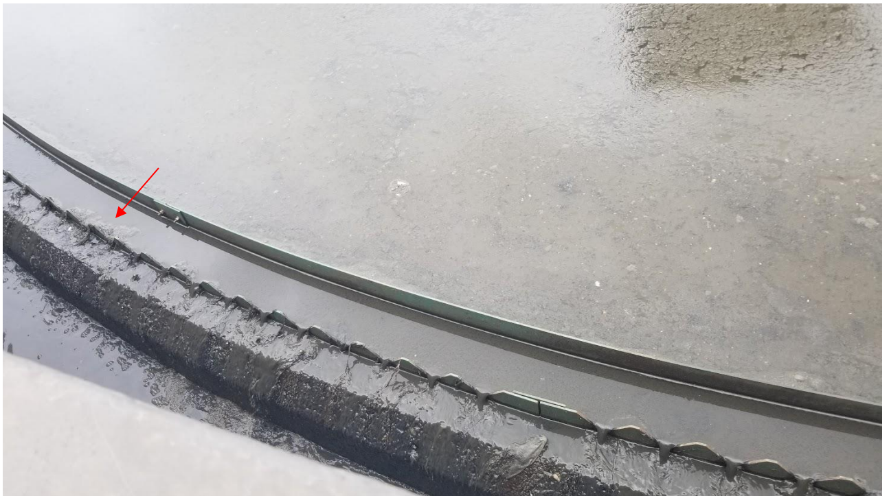
Figure 1d: Close up view of rags and solids next to the V- notch weir (pointed with a red arrow) of GST #2.
