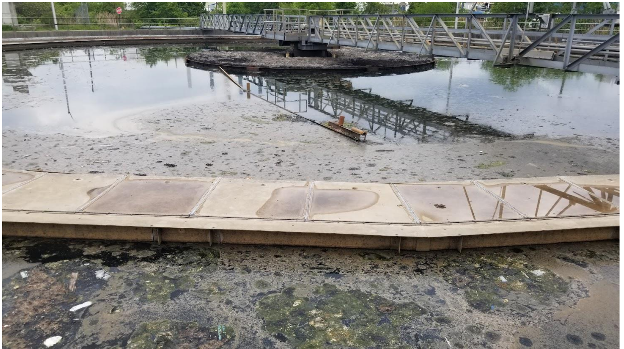
Figure 5h: Scraper arm in Clarifier # 5B. Clarifier # 5B is turned off for maintenance.
