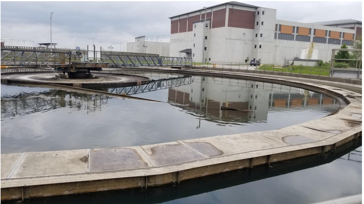
Figure 5j: A scraper arm in Clarifier # 5A is missing.
