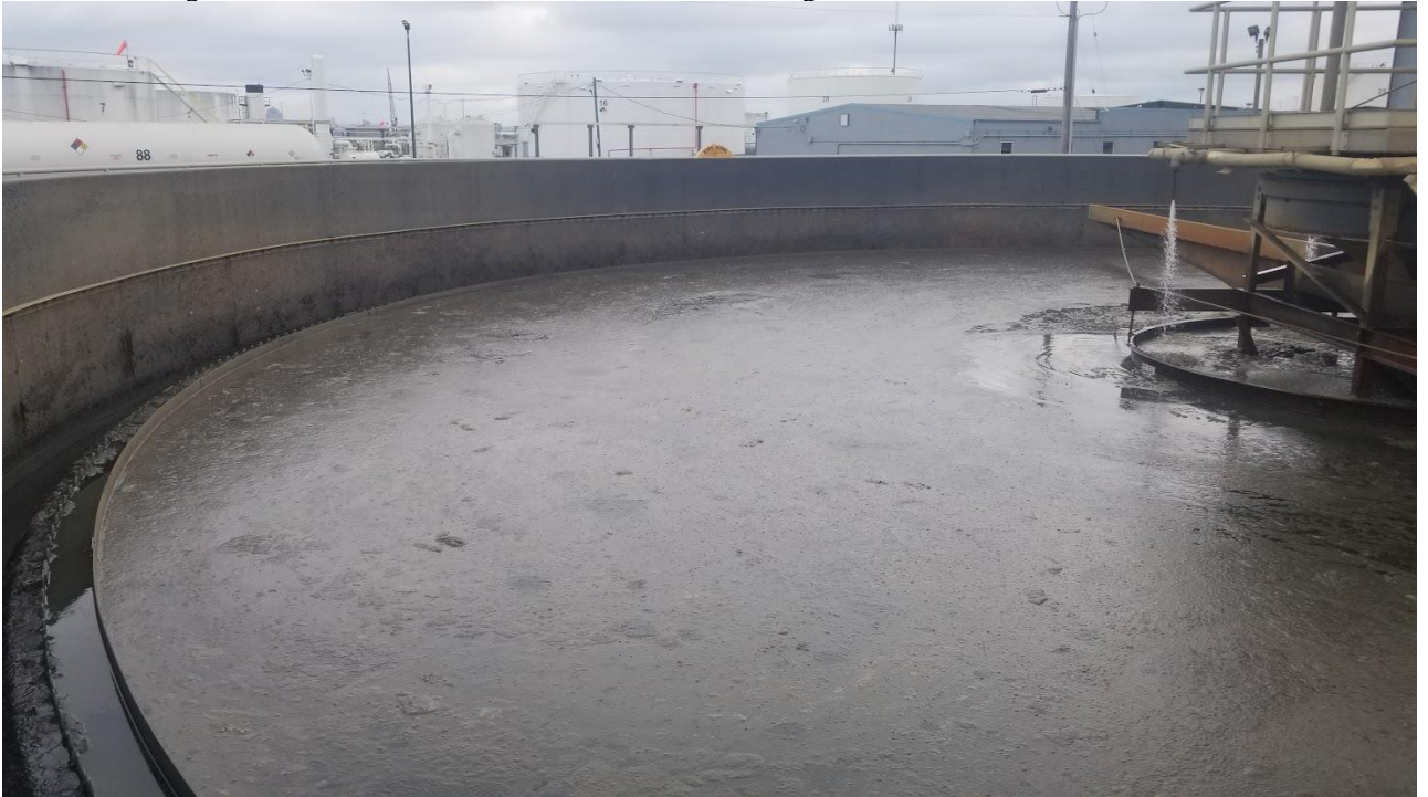
1a: Excessive amounts of sludge at the surface of GST #1. The skimmer arm is above the water surface level.
