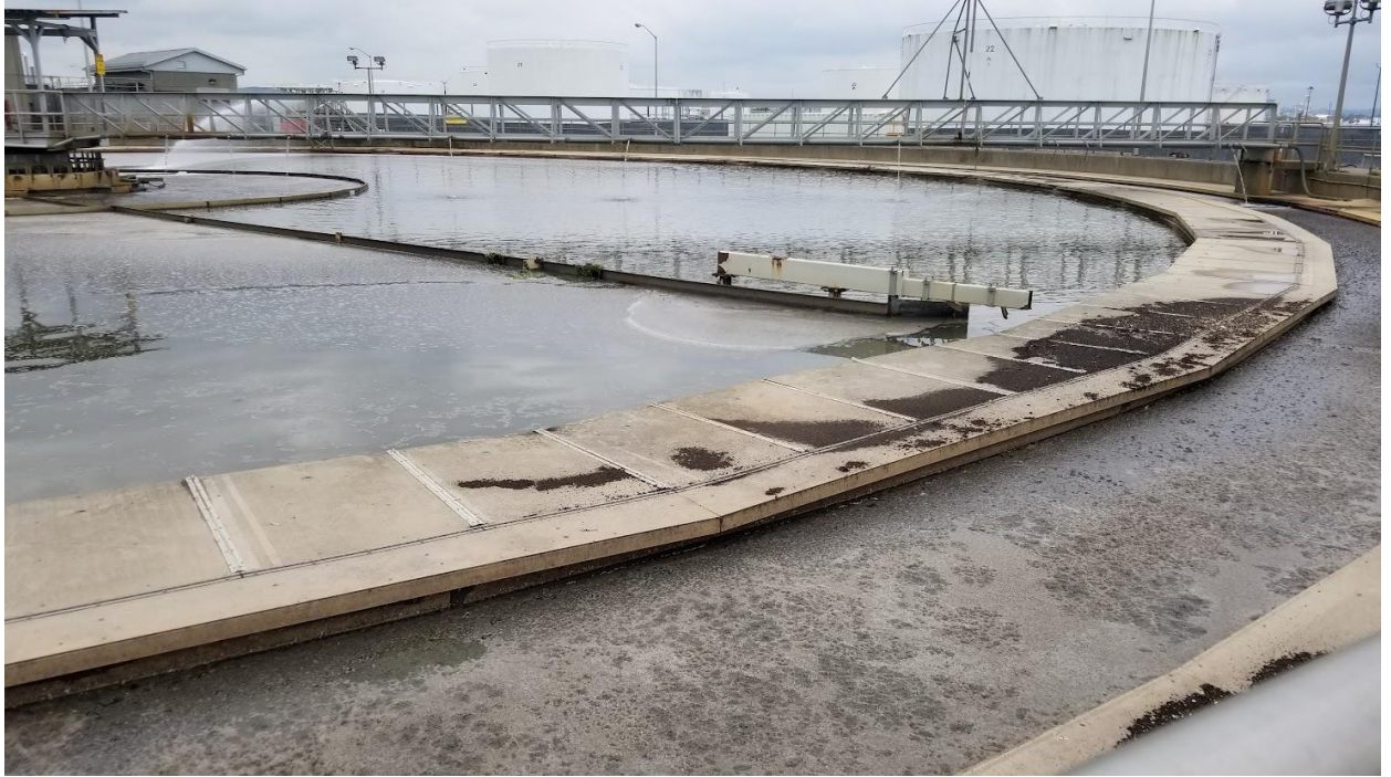
Figure 5a: Rubber part missing at the edge of the scraper arm of Clarifier # 1
