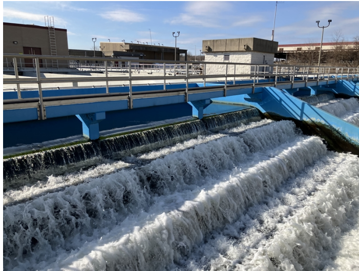
Image 03: Step Aeration system, final effluent.
